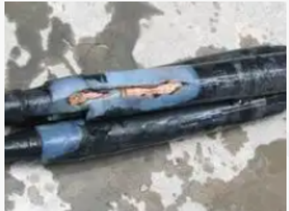
(b) Damp defect
